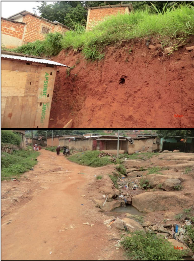
Figure 11. Pictures of eroded land in the city of Danané
